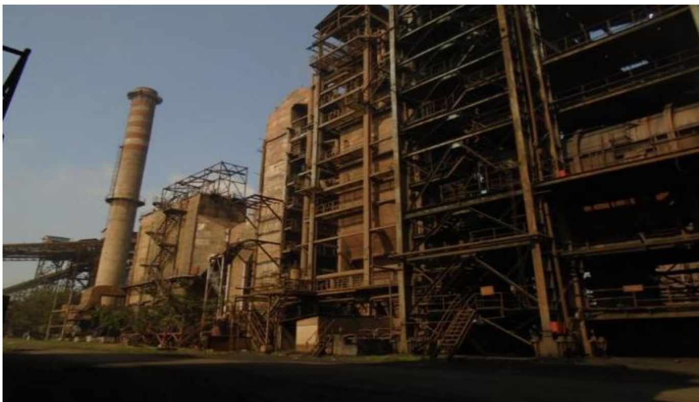
(figure 9: Waste Heat Recovery Boilers)
