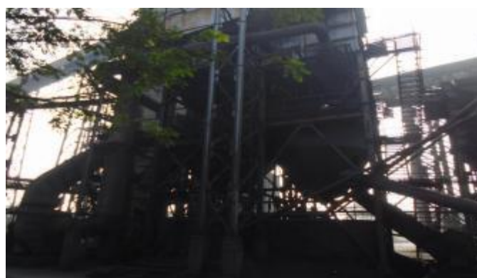
(figure 8: DRI New Bagfilters - Cap:33,200 m 3 /hr)
