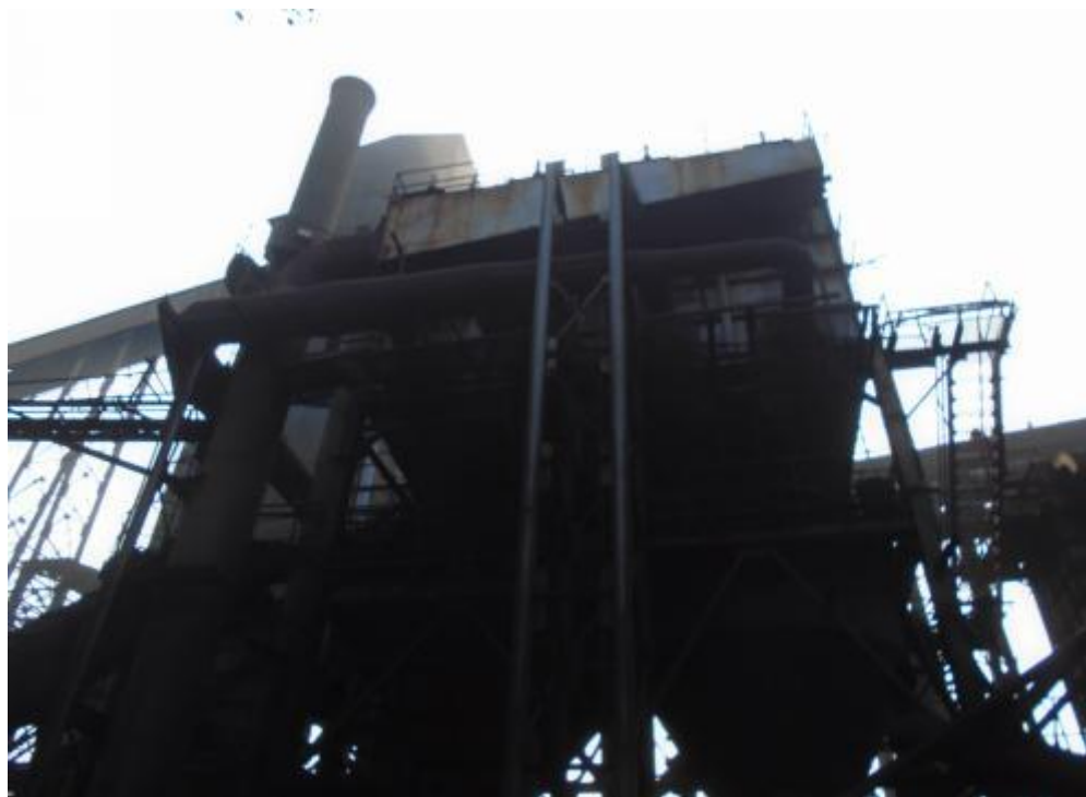
(fig. 8: DRI New Bagfilters - Cap:85,000m 3 /hr)
